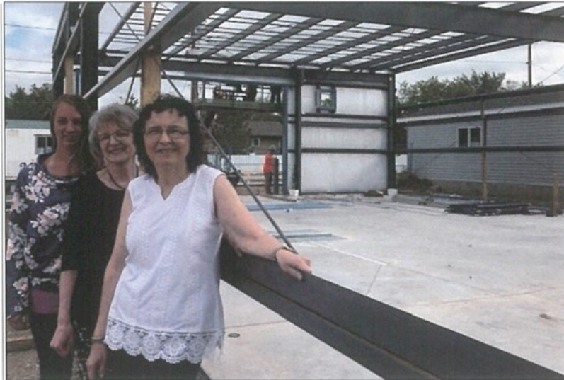
Dundurn Rural Water Utility office staff (L to R) Chantel Hendry, Barb Olyniuk and Ros Arndt are excited about the new building and patiently await for it to be completed.
