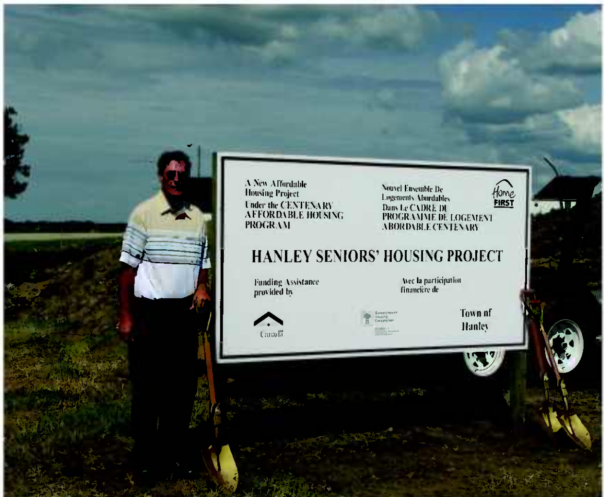
Official Sod Turning in June of 2007. Darryl Grindheim is now the Project Manager for the Saskatchewan Elks Senior Citizens Home in Hanley. It's been a long time, but we are finally done.
